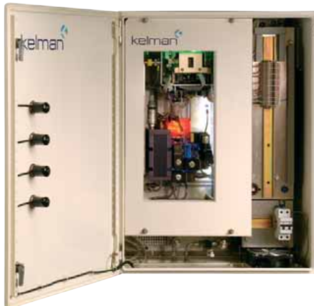
Fig 1 - Inside the TransFix unit.
